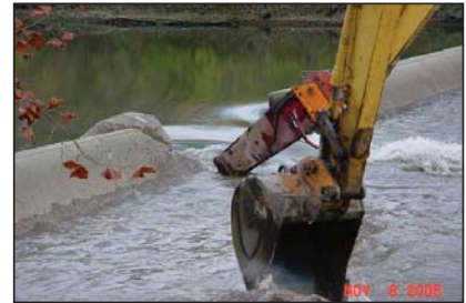
Cutting a notch in the River Street Dam on the Olentangy River
