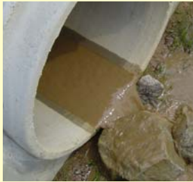
Outlet from storm drain showing soil in run-off
